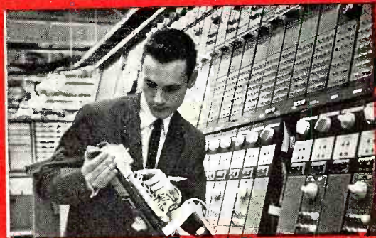
Checking panel wiring of Simplex console
